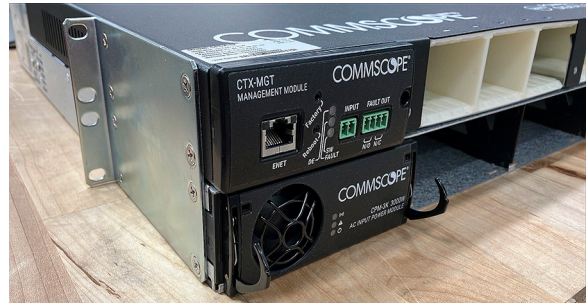
Figure 7. Power Supply in Transmitter
